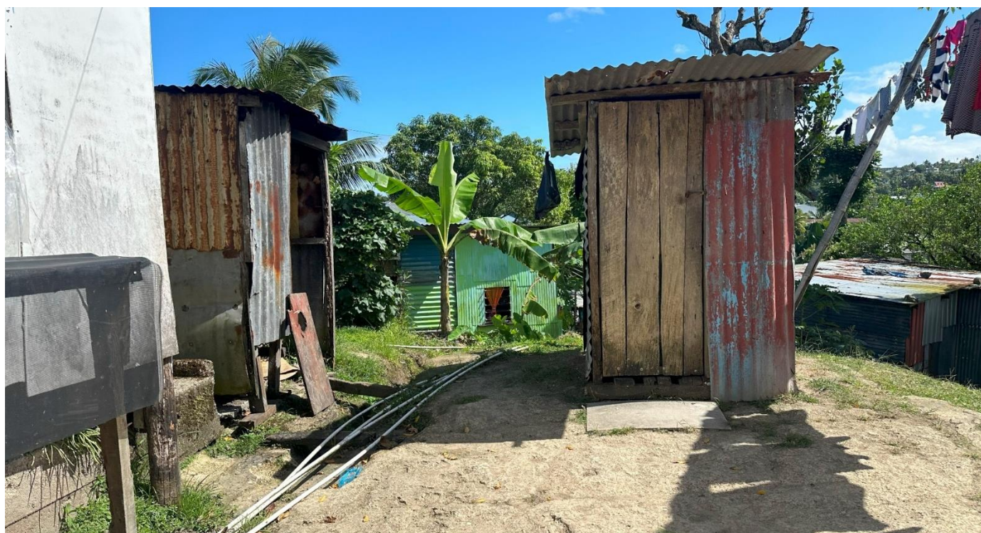
Figure 19: Household toilet and water supply pipes in a settlement in Suva, Fiji (Regina Souter, IWC, 2024)
