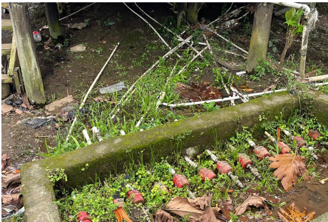
FIGURE 19: CLUSTER WATER METERS AND WATER PIPES INSTALLED NEAR THE BOUNDARY OF AN URBAN INFORMAL SETTLEMENT, SUVA, FIJI. PHOTO: B. ROUSSO, IWC
