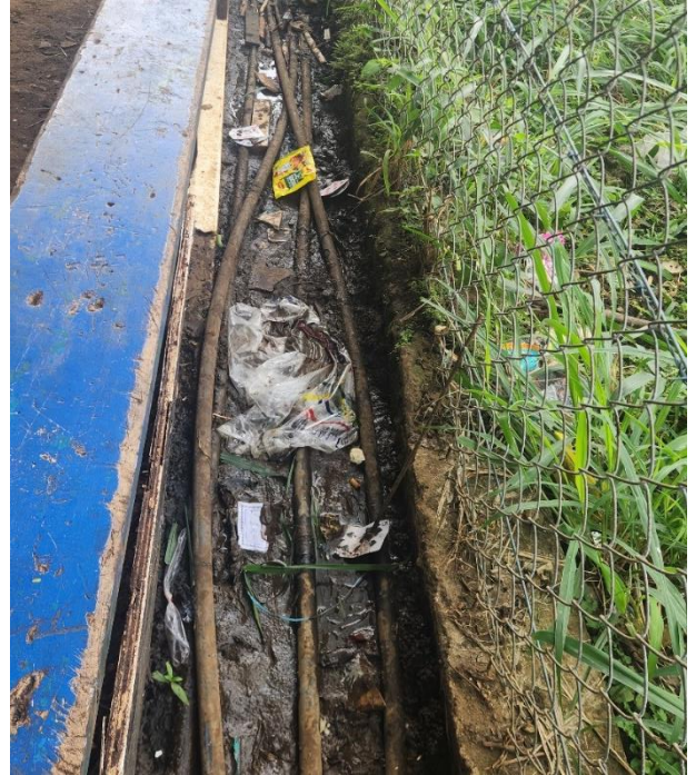
Water supply pipes laid in a drainage channel in an Urban informal settlement, Port Vila, Vanuatu. (R. Sanderson, IWC)
