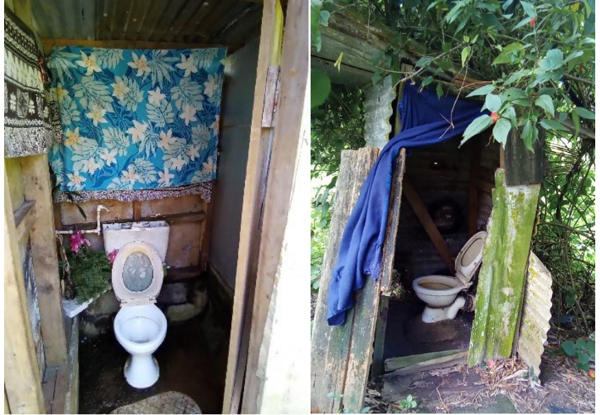
Water-based toilets in settlements in Suva, Fiji (Photo: USP)
