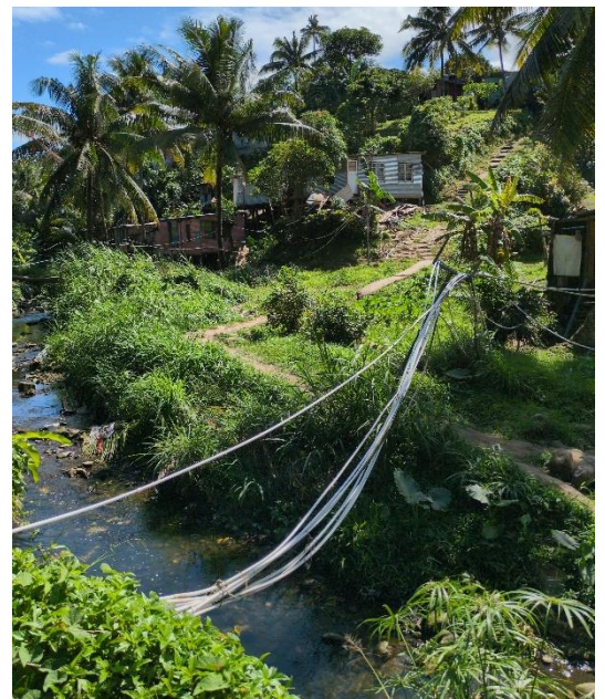
Water supply pipes within an urban informal settlement, traversing a waterway, demonstrating high vulnerability to local flooding and other activities damaging pipes. Suva, Fiji (Souter, IWC)
