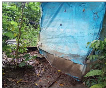
FIGURE 10: SUBSTANDARD SUPERSTRUCTURE MATERIALS
