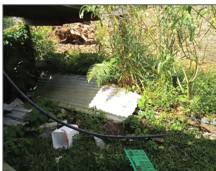
FIGURE 3: EXPOSED WATER PIPES
