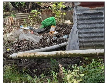
FIGURE 11: EXPOSED SEWERAGE PIPES
