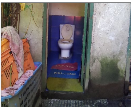
FIGURE 9: SUPERSTRUCTURE AND LATRINE SHOWING WATER LEVEL ENCROACHMENT OF WATER (DARK WATER MARKS ON RIGHT)
