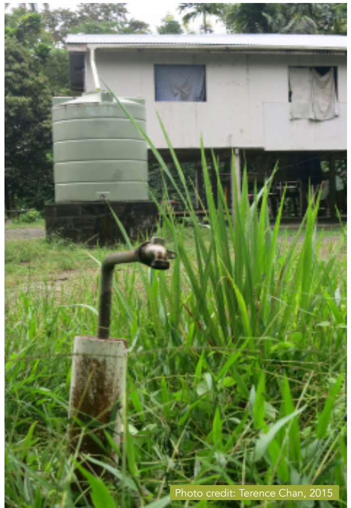
Figure 1: A communal/public rainwater tank in a flood-prone community in the Solomon Islands.
